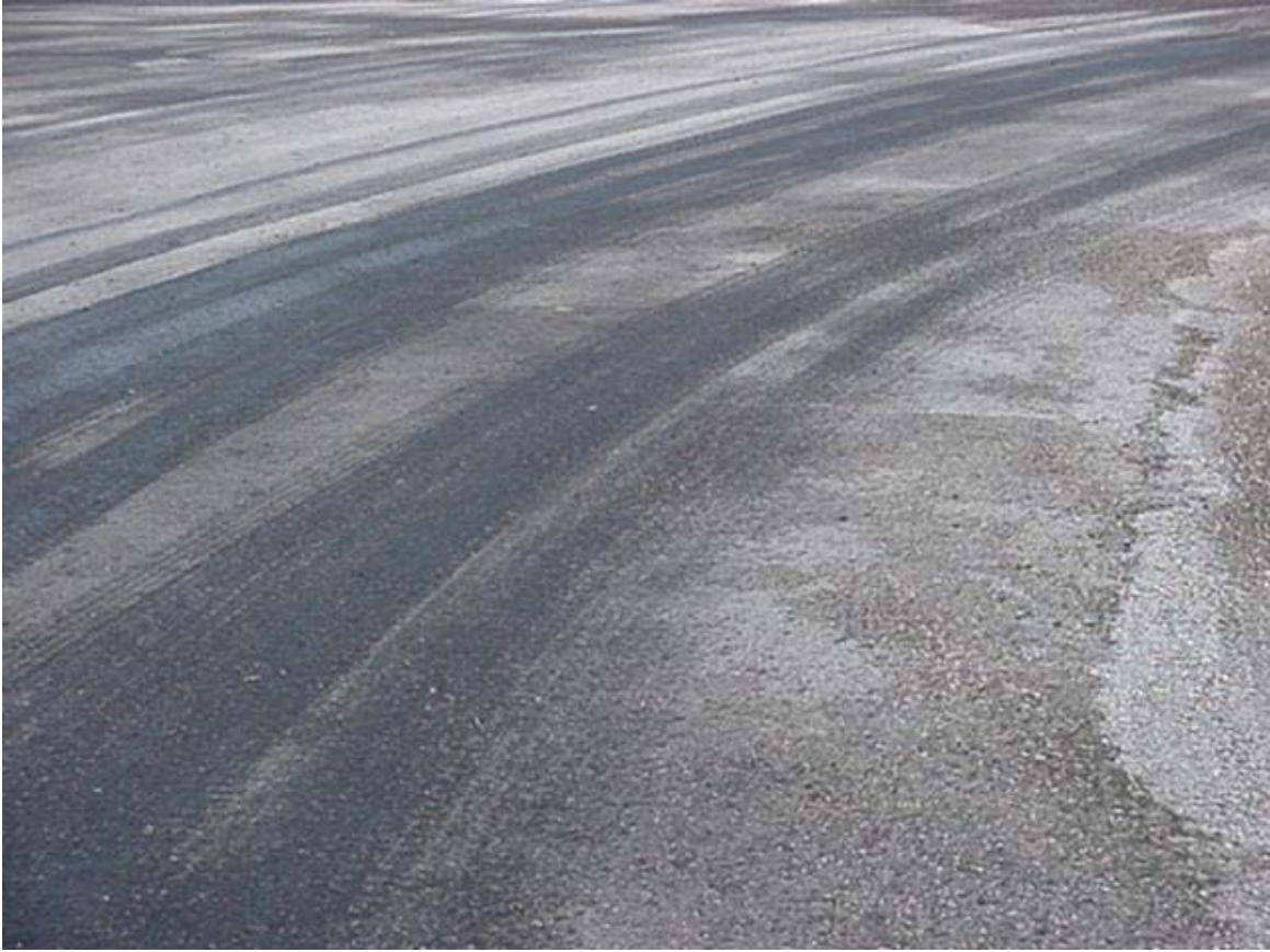
Photo 8. Untreated and icy side road.
