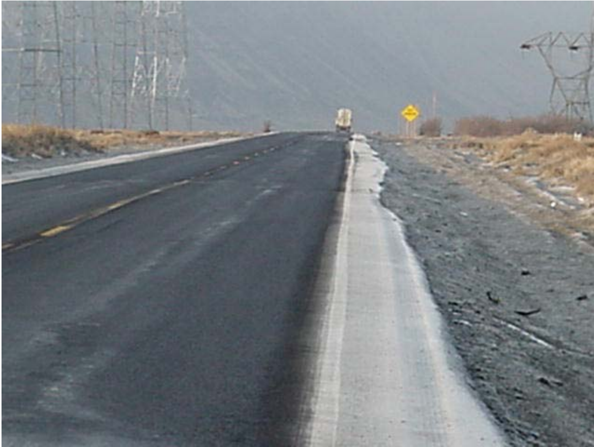
Photo 4. More icy shoulders with bare and wet road. Bare road is due to anti-icing application
