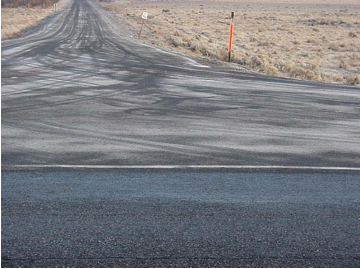
Photo 9. Untreated and icy side road.
